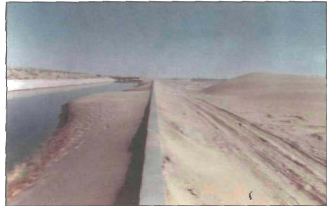
Plate 1. Wind blown sand engulfing IGNP main canal near Mohangarh
